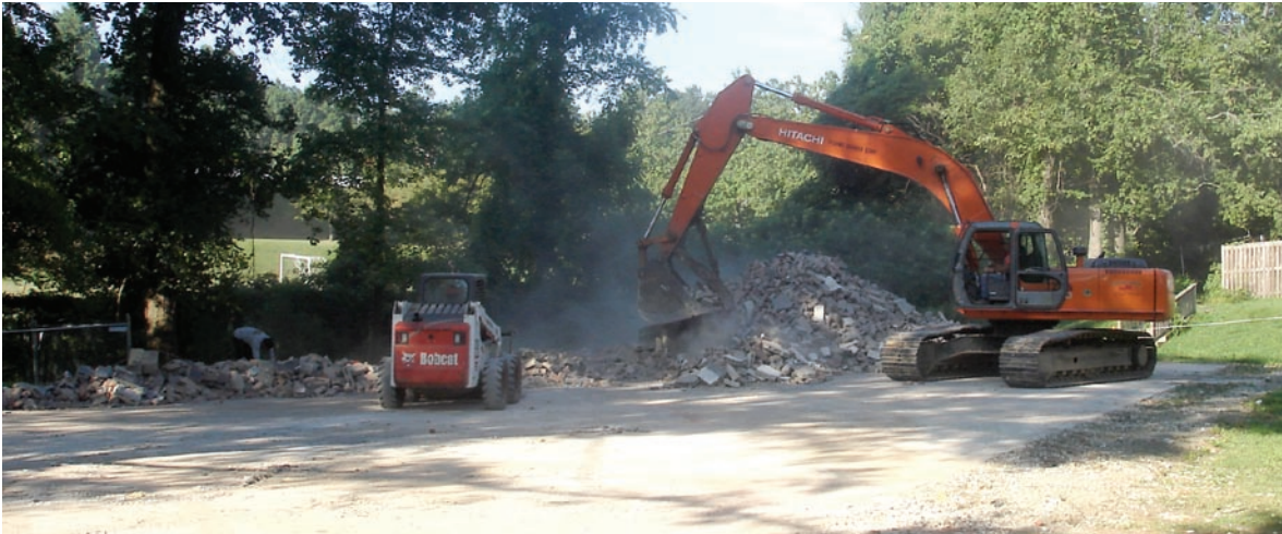
The cleared and prepared site for the future Jeffrey J. Sherman Arts Center
